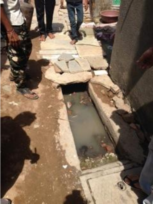
Khodiyarnagar – Open stretch of pipe connecting toilets to the communal septic tank that allows storm water and trash to enter the pipe.
