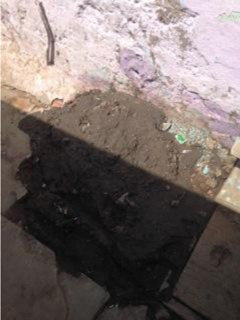
Khodiyarnagar – A pile of human excreta that a resident removed from the pipe connecting toilets to the communal septic tank.
