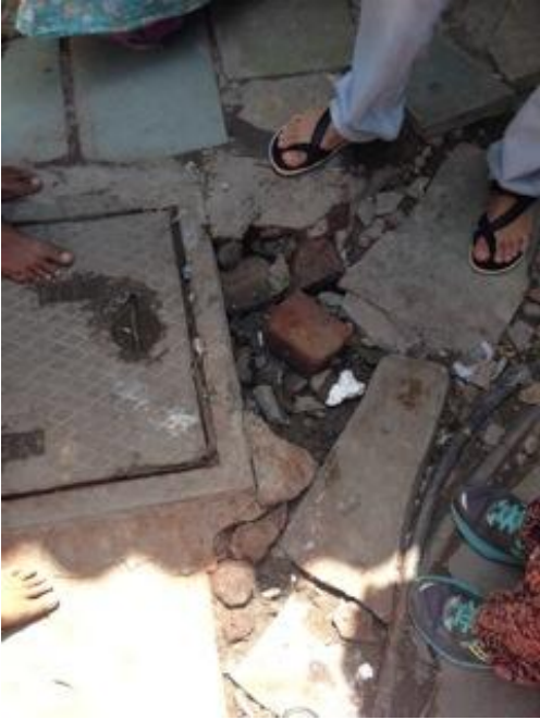
Khodiyarnagar – A broken covering for a manhole, which allows storm water to entire the pipe system.
