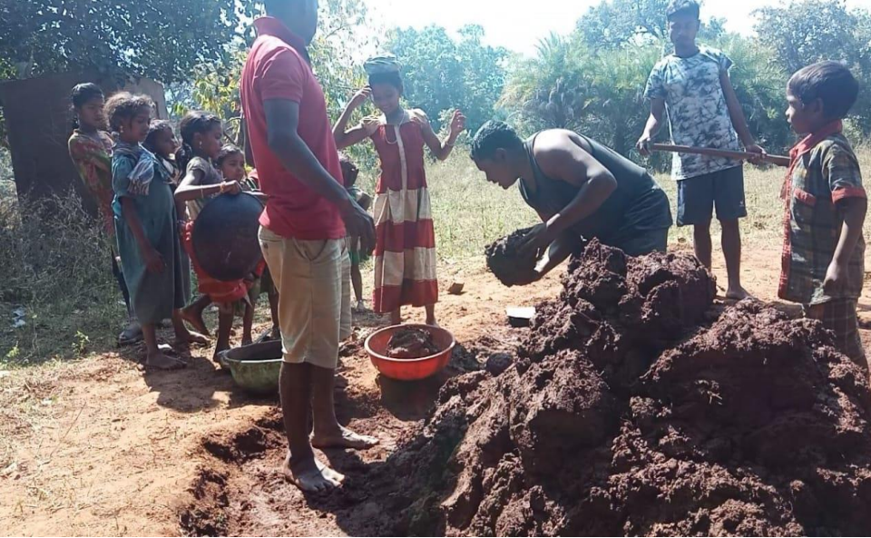
Elders working with youth and children to build their homes using locally available materials .
